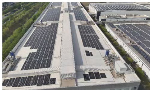
The Distributed PV Project at the Hefei Manufacturing Base
