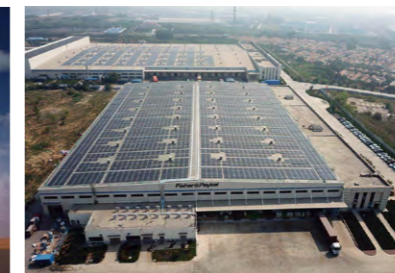
晶澳青岛斐雪派克分布式电站 JA Solar's Fisher & Paykel Distributed Photovoltaic Power Plant in Qingdao
